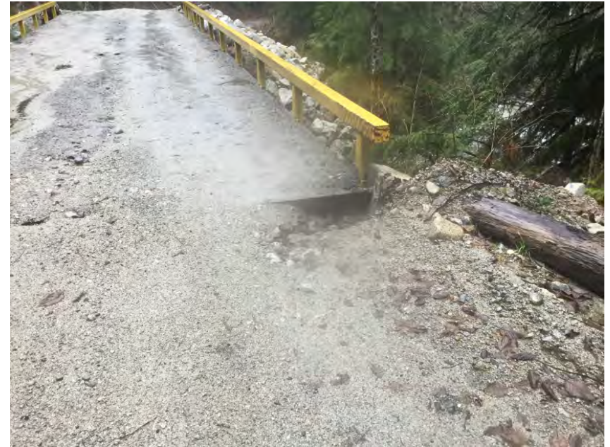
DS right approach losing surfacing material
